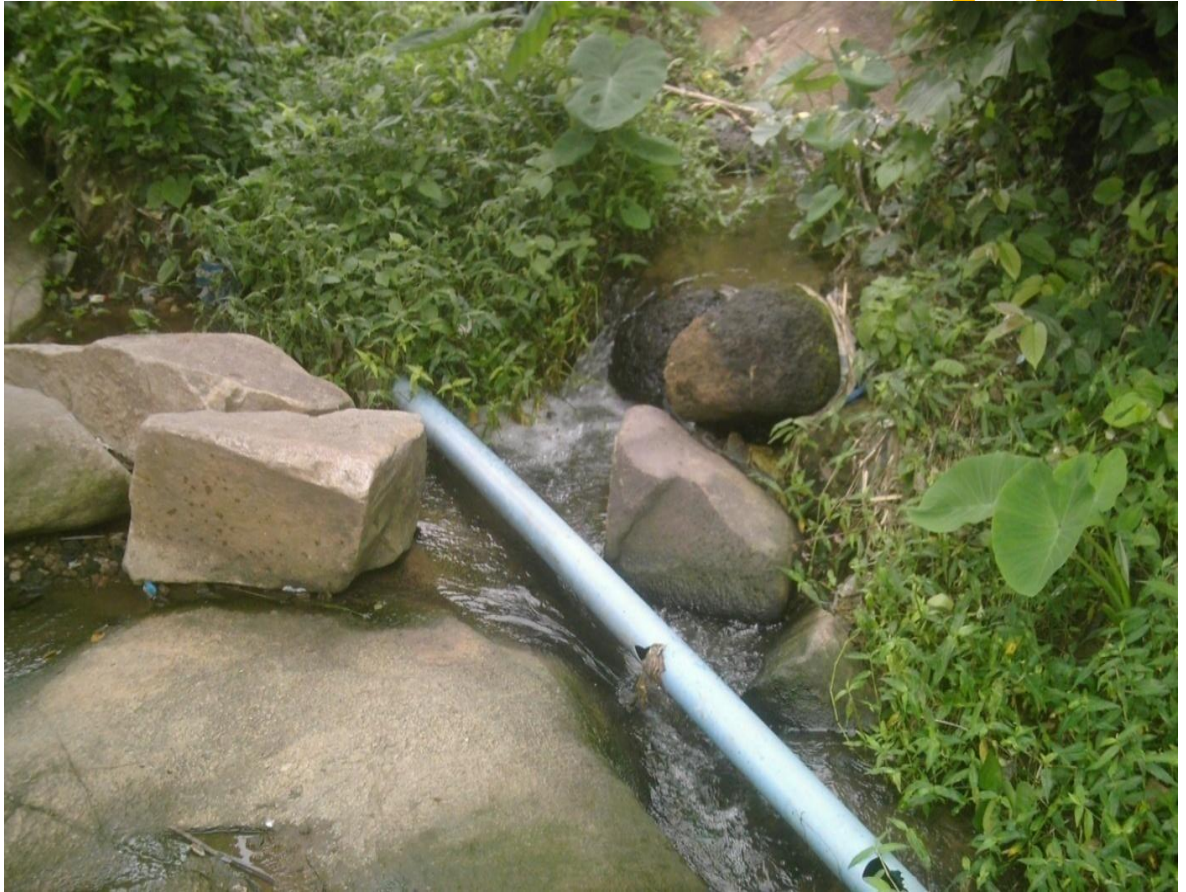
Plate 4.12: Vandalized pipes that carry water from the source to the reservoir
