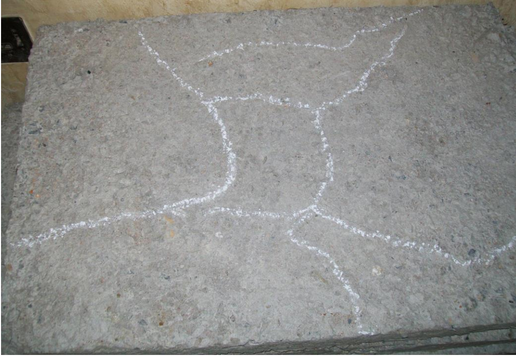
Plate 7: Crack pattern for waffle slab W4 Supported on all 4 sides
