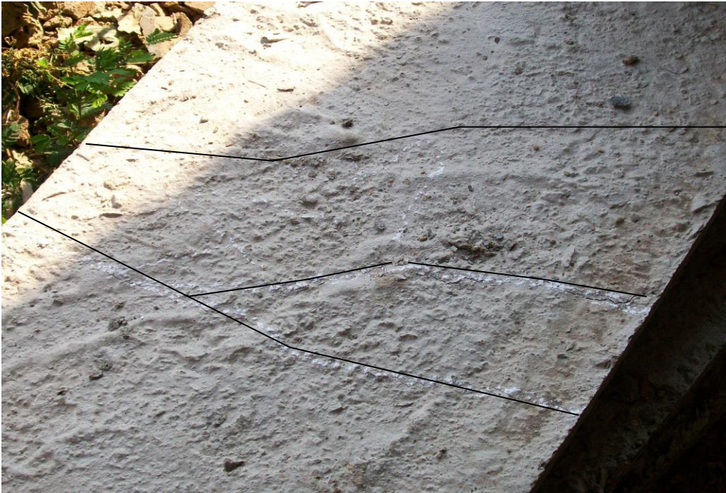
Plate 12: Crack pattern for Solid Slab S6 supported on 1 long side and 2 short sides
