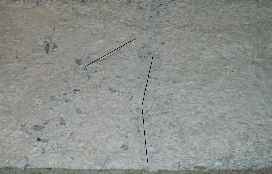
Plate 5: Crack pattern for waffle slab W1 supported on 2 short sides
